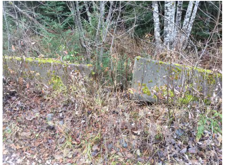
Disconnected transition at downstream right bank
