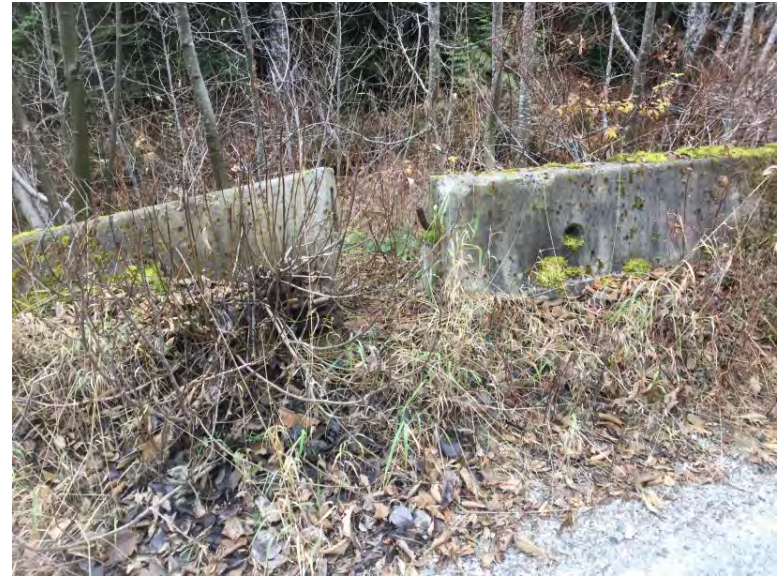
Disconnected transition at downstream left bank
